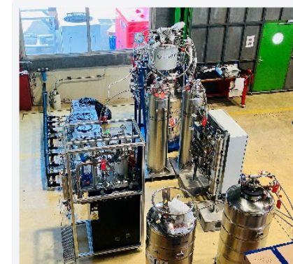
He/H 2 Liquefier & cryostat down to 4K
